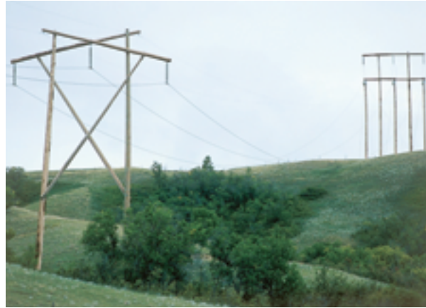
Maintaining vegetation around power lines helps to ensure their safe operation.
